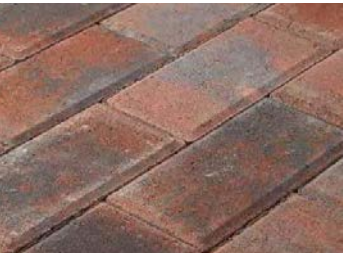
HOLLANDSTONE PAVERS AT SIDEWALKS
